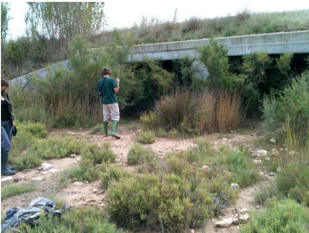
Figure 7.3. Entrance to large multiple box-culvert underpass in Parc Natural deis Aiguamolls de l'Empordia, Cosa Brava, eastern Catalonia, Spain. This underpass is used daily by large numbers of wild boar, as well as numerous other local mammal species. Although the floor of the culvert was originally concrete, this has now been covered in silt. Although no plants grow inside, the natural vegetation on either end is continuous with the surrounding habitat.
