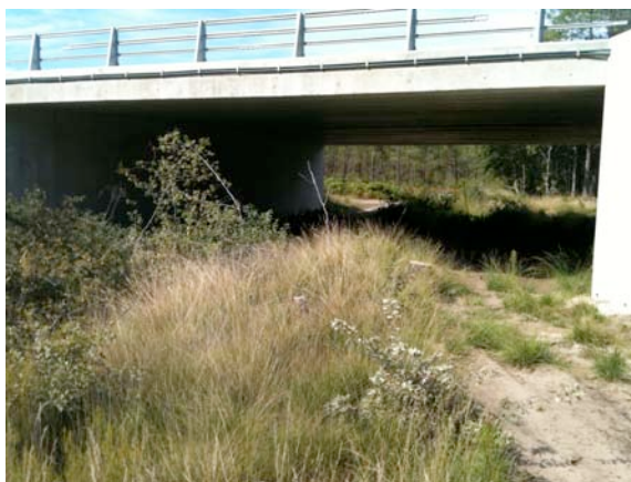
Figure 6.4. Avoidance bridging on C37 motorway in southern France designed to enable complete avoidance of Natural 2000 watercourse site harbouring European mink.
