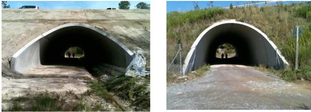
Figure 7.4. Two large ovoid underpasses, with about 3.5m clearance. This design can bear considerable pressures. The structure to the left (southern France) is targeted on roe deer and also allows passage of a small stream. The structure shown to the right (eastern Spain) is also used by roe deer but is strongly co-use, being used by local farmers as well as recreationalists.
