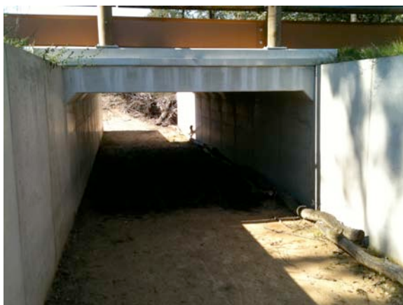
Figure 7.5. Floor of recently constructed box culvert underpass showing sand/earth surface and habitat logs (The Netherlands)
