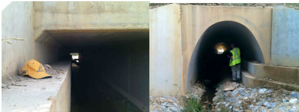
Figures 7.6. Examples of solid ledges incorporated into the walls of two different underpasses in southern France.
